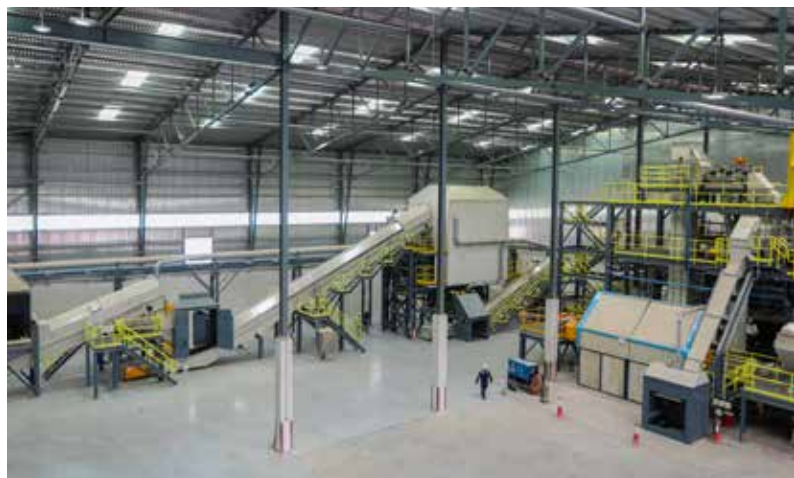
Despite COVID-19 challenges, the SPL Treatment Plant Project achieved more than 750,000 Safe working-hours w/o LTI © Alba
